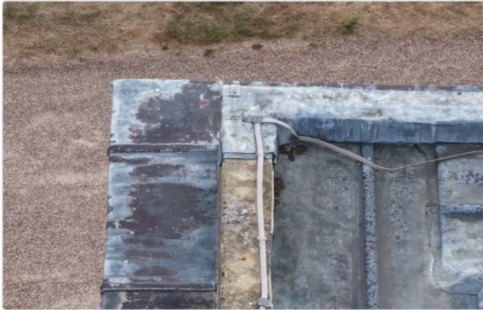
D02-A — Blocked Gutters / Outlets, Gutter Line
