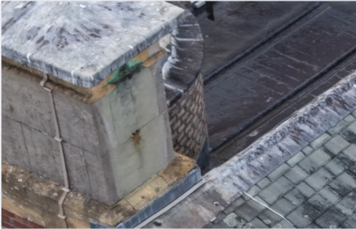
D03-A — Chimney / Stack Deterioration, Around Chimney / Stack
