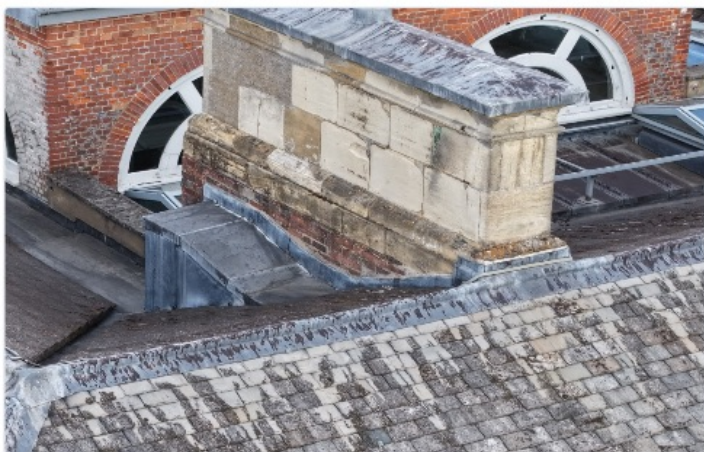
D04-A — Chimney / Stack Deterioration, Around Chimney / Stack
